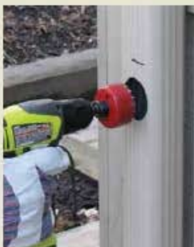
Drill hole in downspout
